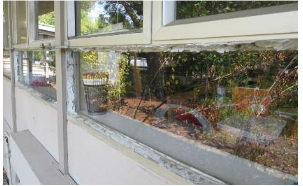
Deteriorating window casing at one Lafayette school.
